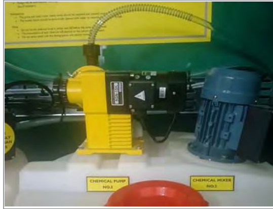
2 Automatic Chemical Mixing & Dosing System
