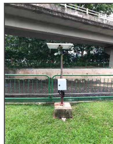
Typical CCTV Installation with Solar Panel on top
