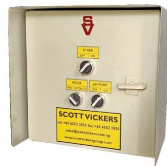
Control Panel for Mixer & Dosing System
