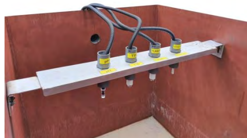
Monitoring Probes in Collection Tank
