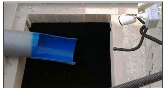
Typical CCTV Installation adjacent to public drain
